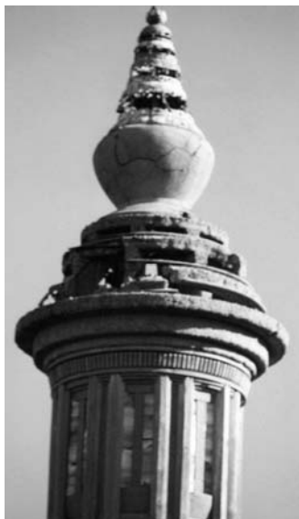
close-up of finial on smoke stack minaret of power house pictured above
